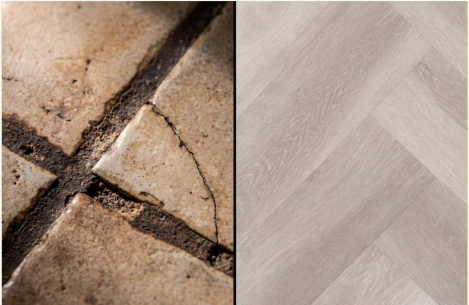
Cracked, stained grout (tile) vs continuous seamless surface (Glue-Down SPC)
